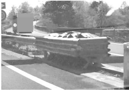
Deformed absorber at accident spot
