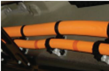
Figure 7. HV-lines with orange warning colour
