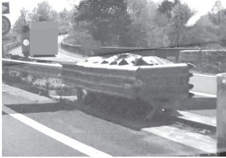
Deformed absorber at accident spot
